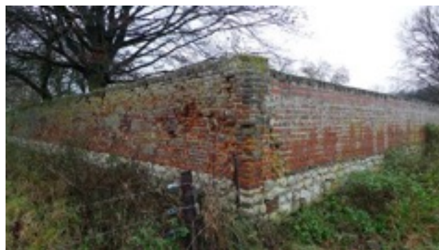
Fig 7: the south wall from the same place as Fig 6 but around 60 years later. Picture © Wade Krawczyk
